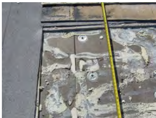
Fig.3. Soft, off ratio foam adhesive with no body, poor bonding
